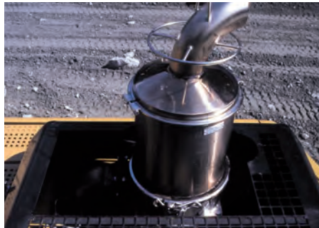
Figure 20 : Use of particle filters is part of the concept for environmental protection (© AlpTransit Gotthard Ltd)
