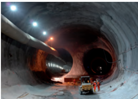
Figure 4 : - Top: Drilling jumbo working in a conventional tunnel drive. - Below: Tunnel bifurcation excavated by conventional tunnelling General description of the project development process © AlpTransit Gotthard Ltd.
