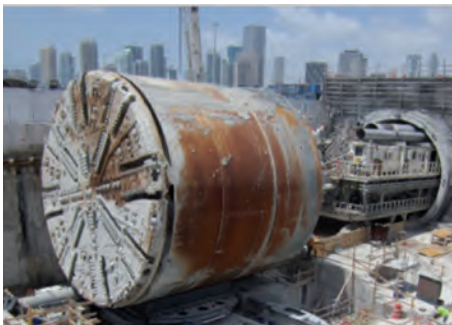
Figure 2 : Top left: Lowering a TBM into the start shaft Lower left: TBM arrived at the portal with back-up still inside the tunnel © Babendererde Eng
