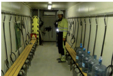
Figure 19 : Modern refuge chamber ® ATG
